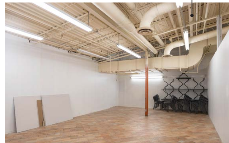
Easily accessible ventilation system
