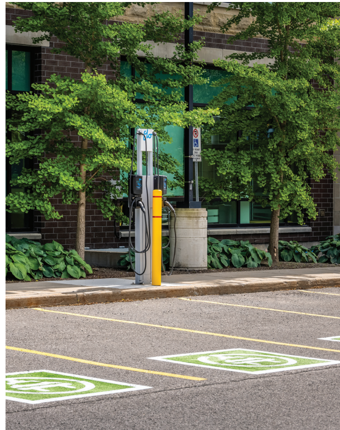
EV charging stations installed in 2023 2611 Queensview Drive, Ottawa, ON
